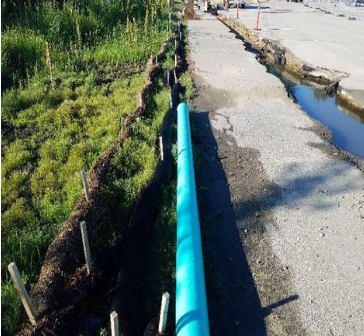
Fig 9: Straw wattle and sock installed in low lying area in "A" lot, next to trench. Viewing south. (7-01-19).
