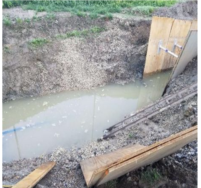
Fig 12: McCourt is pumping water out of trench along Colovos Rd. Viewing west. (7-01-19).
