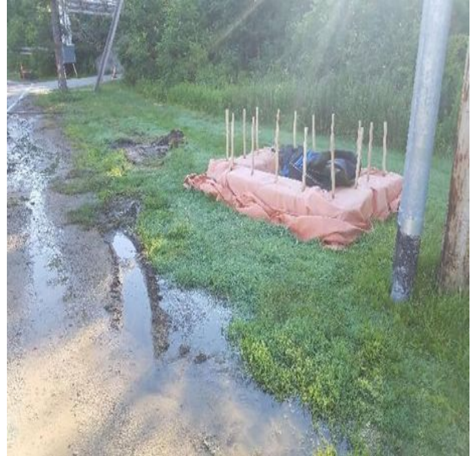
Fig 10: Dewatering apparatus next to Colovos Rd. McCourt has been pumping storm water out of trench. Viewing northwest. (7-01-19).
