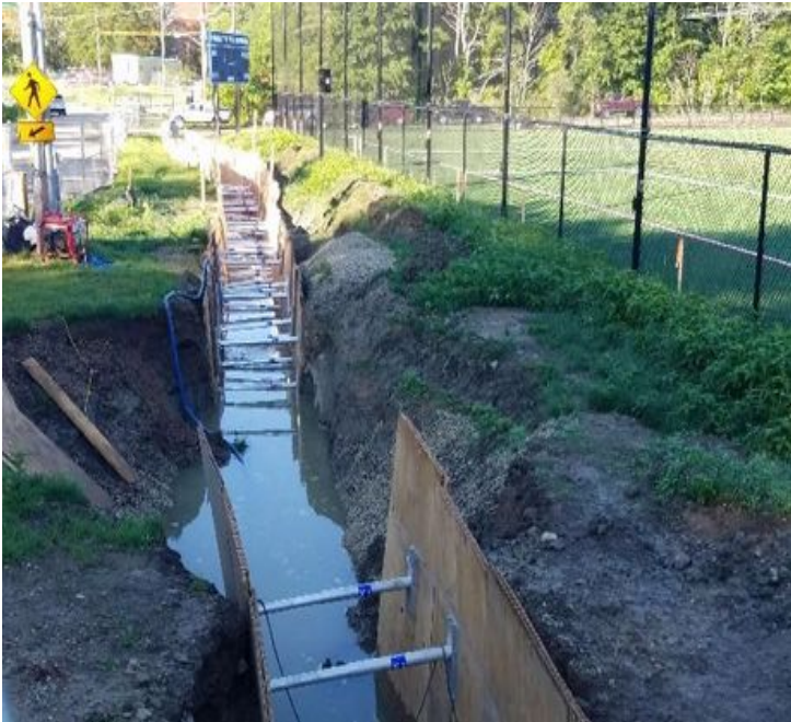
Fig 13: Rain water in trench along Colovos Rd. Viewing south. (7-01-19).
